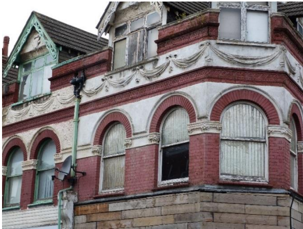
Poor condition of upper levels of some buildings
