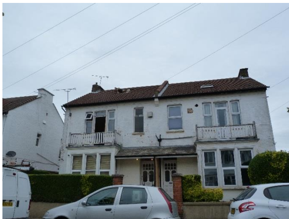
Poor decorative condition of houses on Ditton Court Road, together with inappropriate alterations such as uPVC windows
